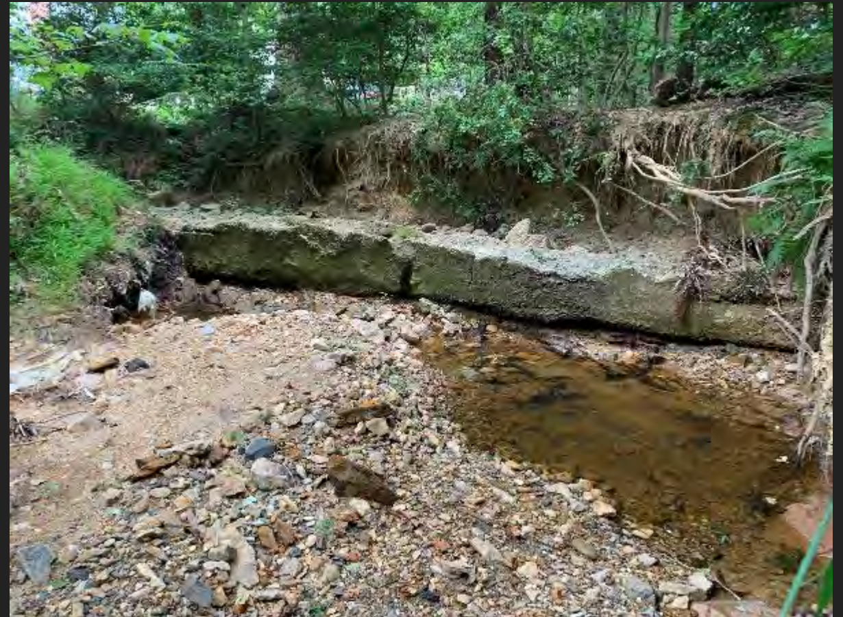
Urban Stream Syndrome: Eroded channel and exposed sewer line at Trapp Rd, Annandale, VA
